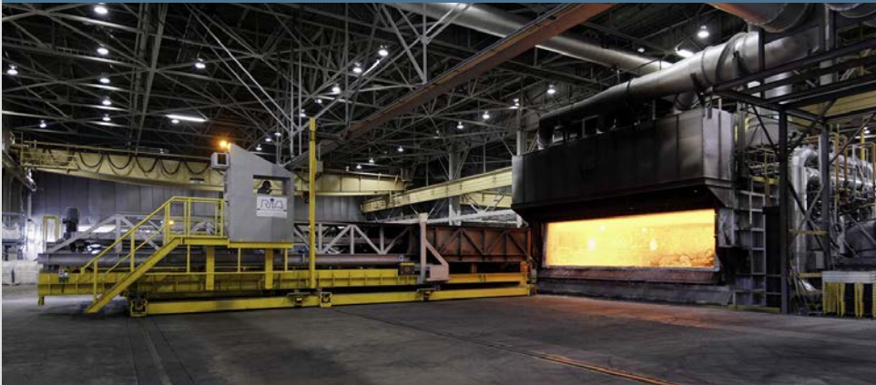
Front load melting furnaces and charge cars at our Kalamazoo casting facility conserve energy by reducing heat release.
